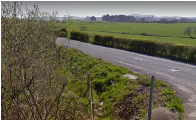
Photo Left. Junction of New Line Road and Killeenan Road looking southeast. Roadside drain running down New Line Road with culvert under Killeenan Road.
